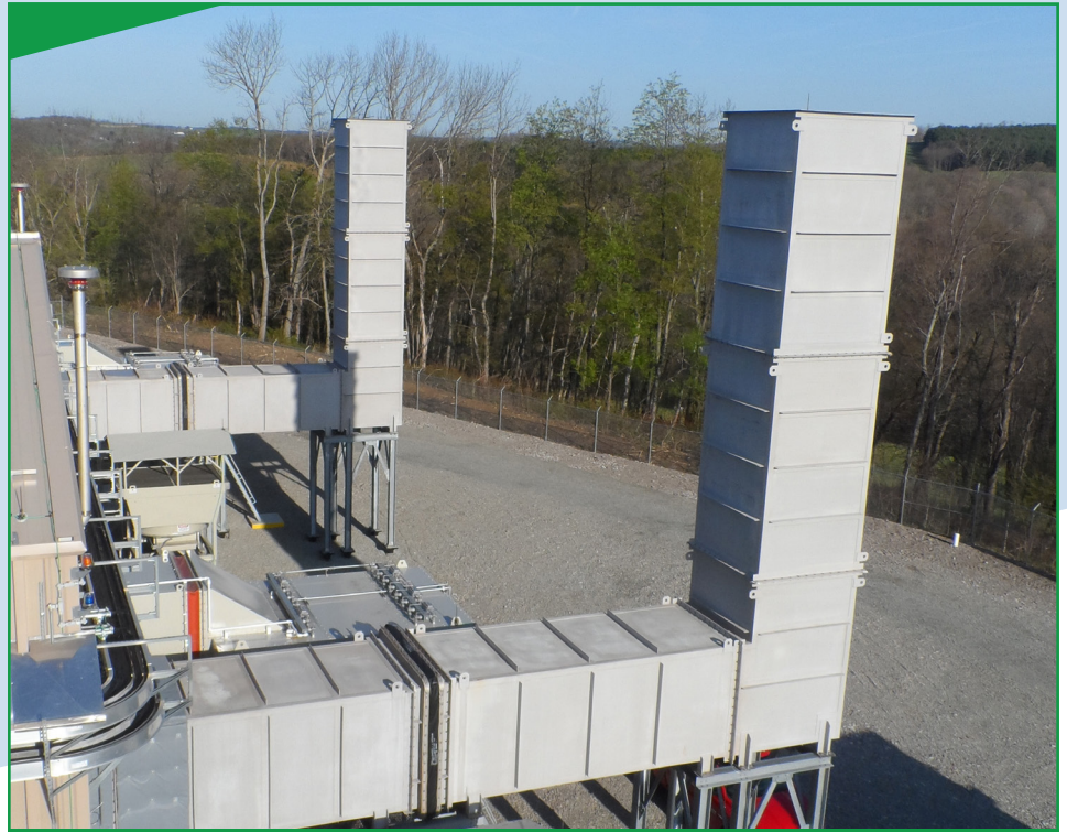
Turbine Ducting Systems
