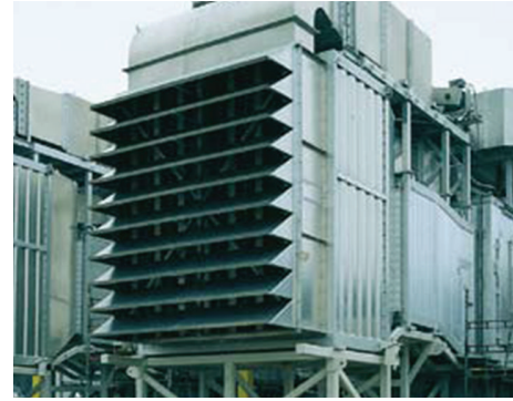
FIGURE 4: Weather Hood on inlet filtration system [34].
