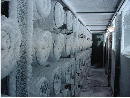
FIGURE 5: Pulse cartridge filters with frost build up due to cooling tower drift [29].
