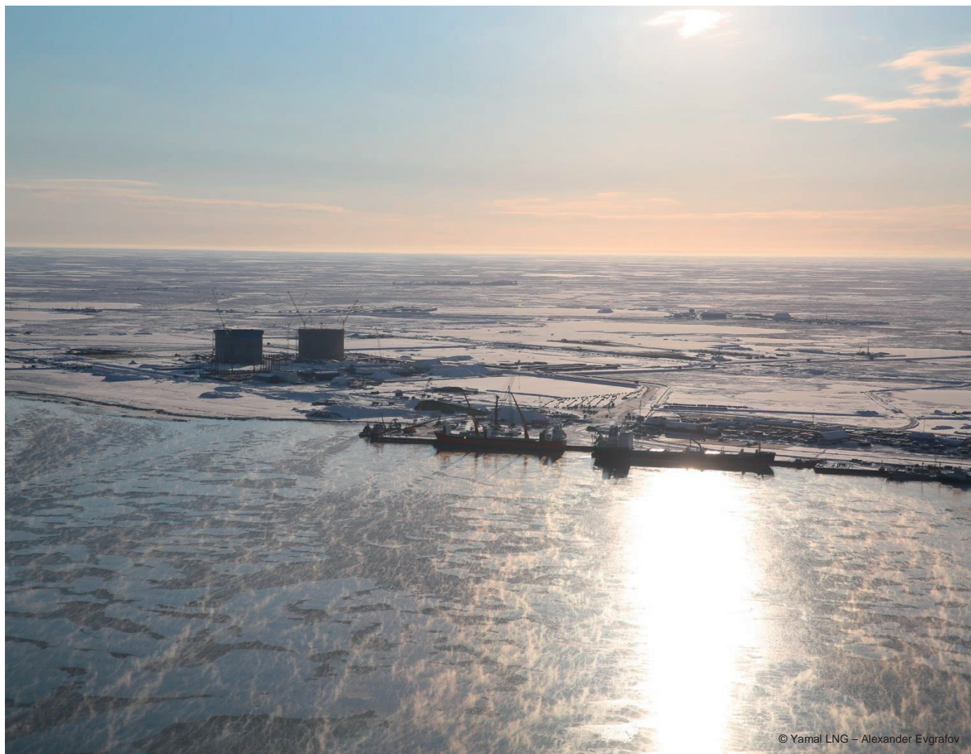
The 16.5 MTPA Yamal LNG project being executed on the Yamal Peninsula (Russian Federation) beyond the Arctic Circle with start-up slated for 2017 (first train), 2018 (second train), and 2019 (third train)
