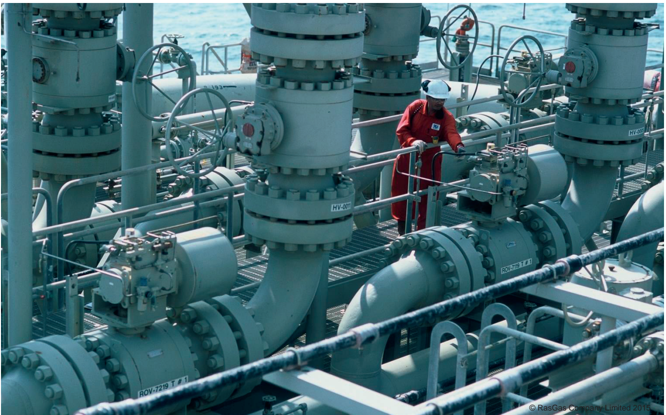
RasGas Employee Inspecting Offshore Riser Platform Drain Manifold
