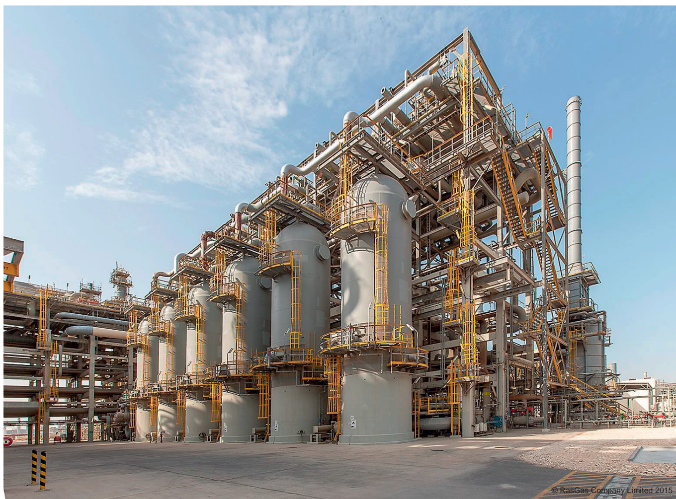
Ras Laffan III Trains 6&7 Dehydration Units
