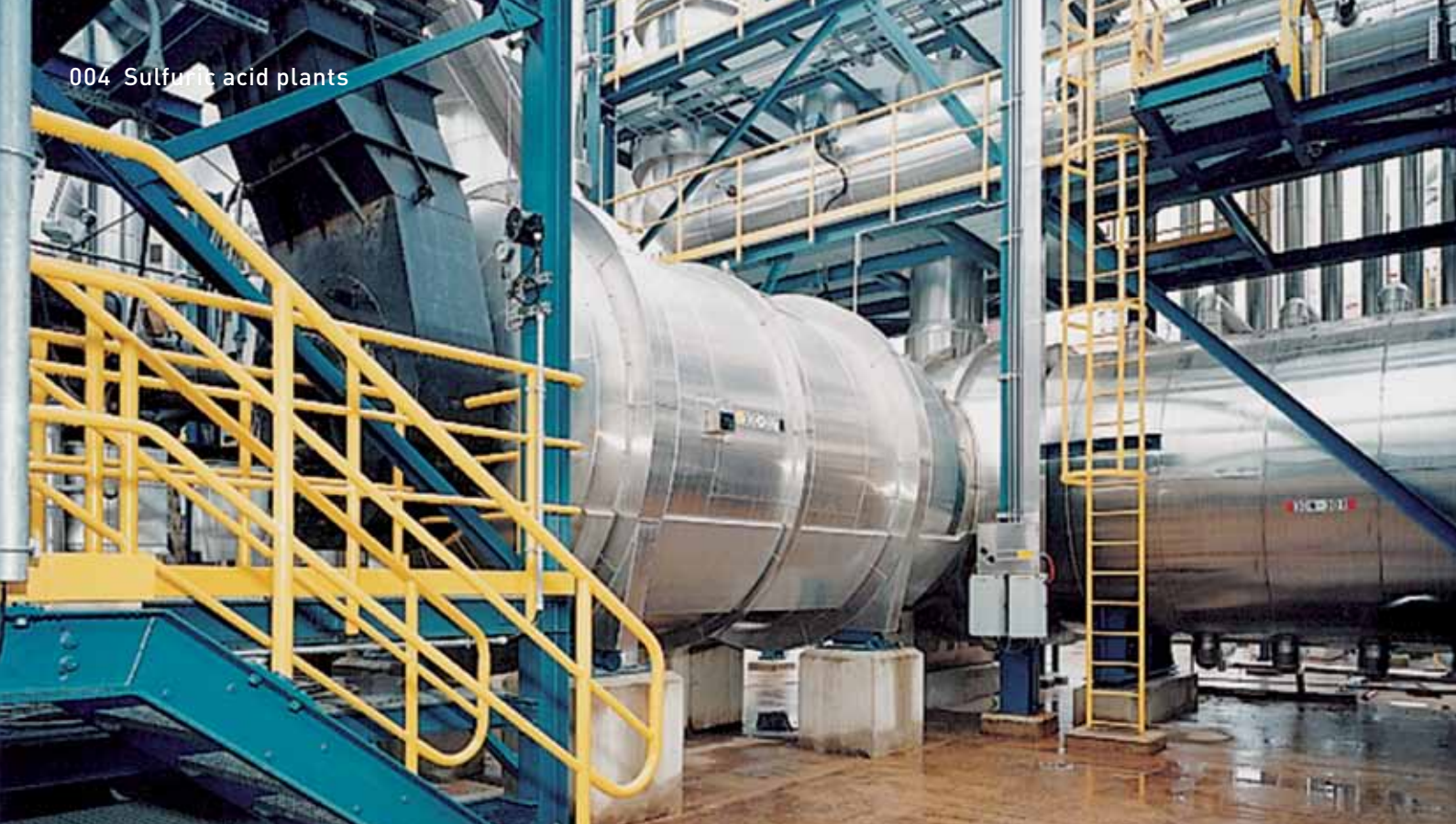
Sulfur combustion furnace and fire tube boiler.
