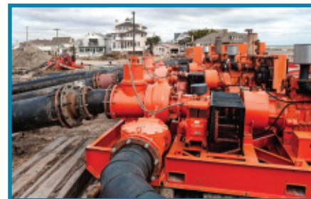
In the immediate wake of Hurricane Sandy, Xylem pumps and analytical instruments were deployed in hard-hit locations. Above, our Godwin dewatering pumps remove sea water from a flooded area near Belmar, New Jersey, and return the water to the ocean.
